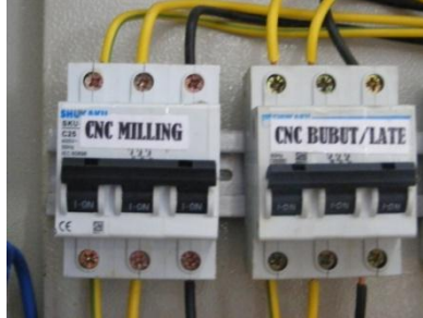
Gambar 3. Main Switch Posisi ON
