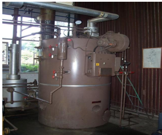
Gambar 1. Oil Fired Boiler Fulton Type E30
