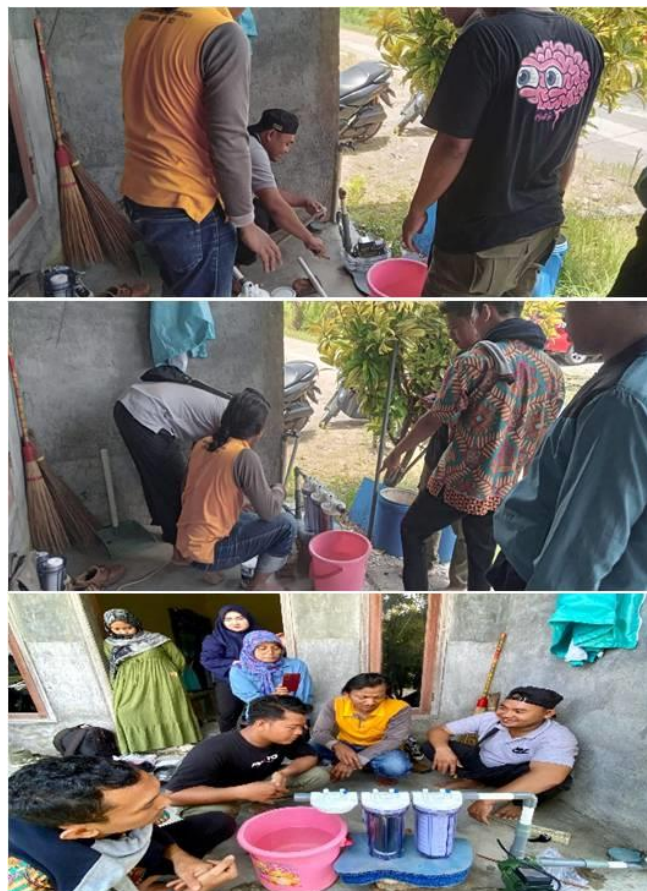
Gambar 4. Instalasi Alat Filtrasi model PWC-FG
